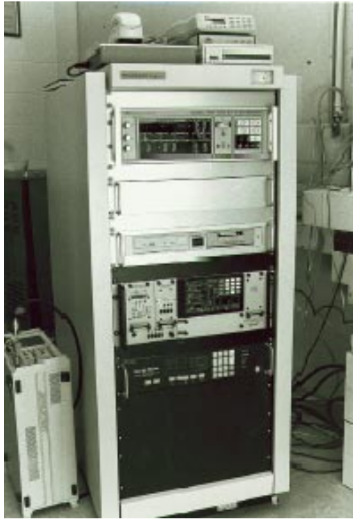
Fig. 5. The 1.2-m LEO-D terminal rack housing the control workstation, communications interfaces, antenna controller, and the entire receiver.
