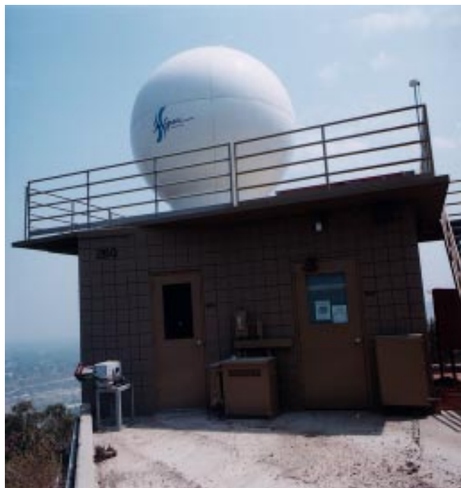
Fig. 4. The LEO-D radome/antenna assembly installed on Building 260 on the JPL Mesa during SAMPEX and EUVE demonstrations. (The assembly was moved to the rooftop of Building 238 in April 1995).
