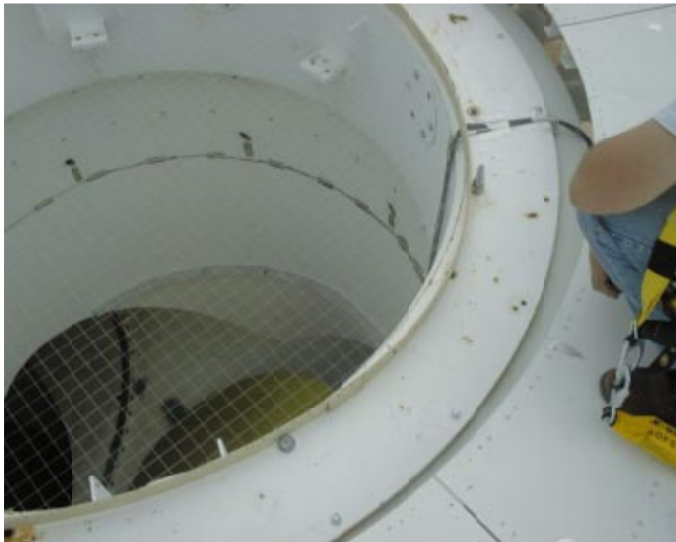
Fig. 2. A bird's-eye view of the installed bird net.
