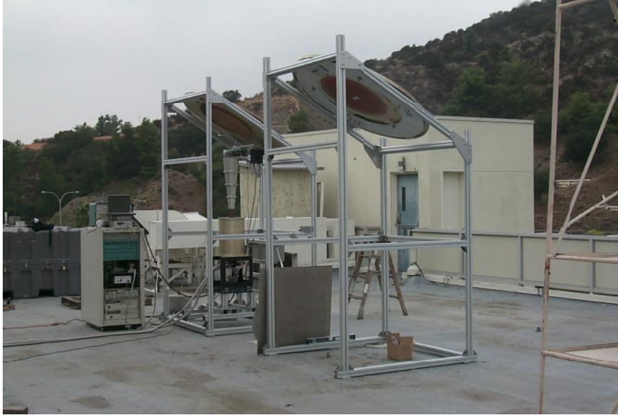
Fig. 1. View of the test setup on the roof.
