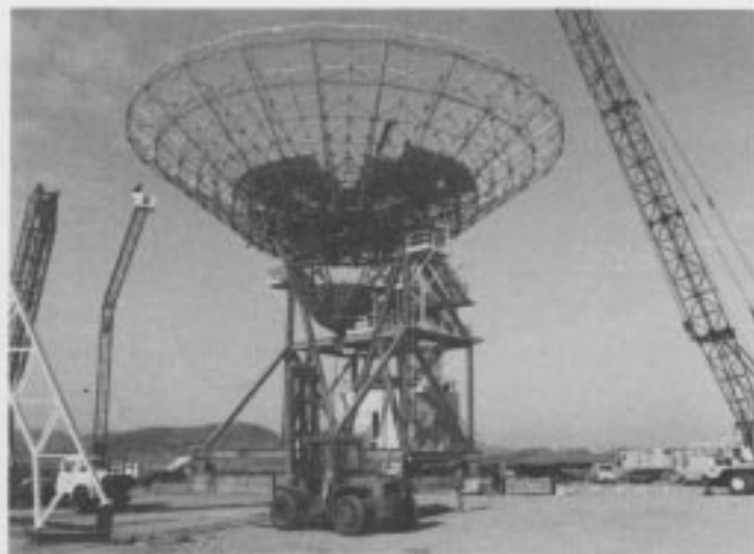
Fig. 10. Reflector and panel support, DSS 15
